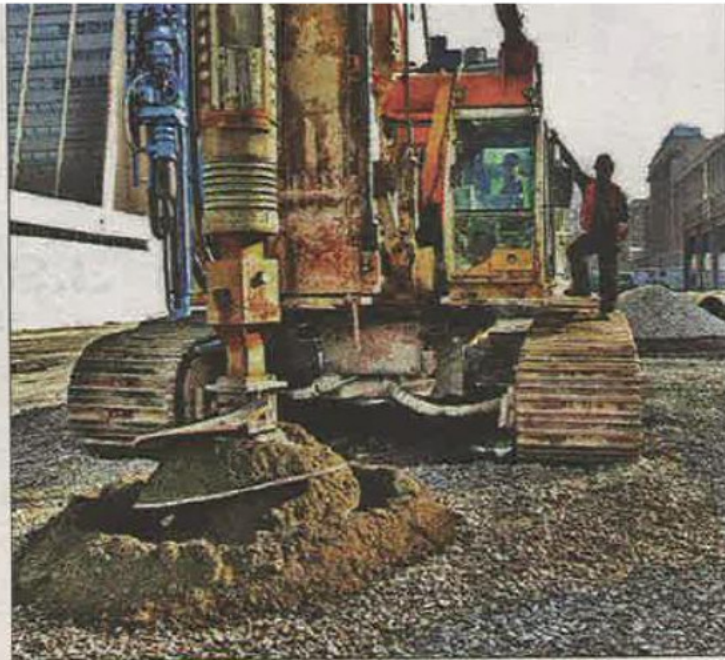
A giant drill rig breaks ground on the Hudson Yards construction project December 4, 2012.
