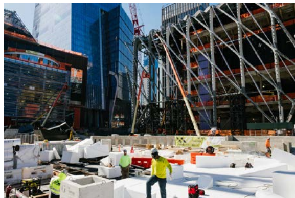
Hudson Yards Centerpiece Begins to Rise The Culture Shed (right) with 10 Hudson Yards (center) and the shopping center.
