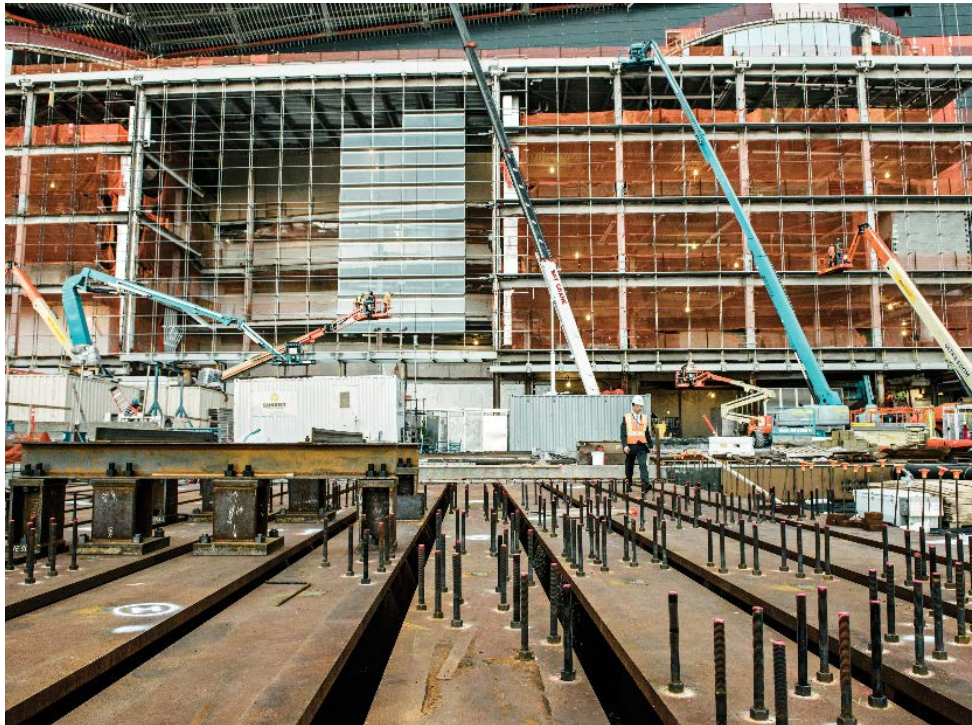
The foundation for Vessel, the centerpiece installation of the public square and gardens, with the retail complex behind it. Photo courtesy of Joshua Scott
