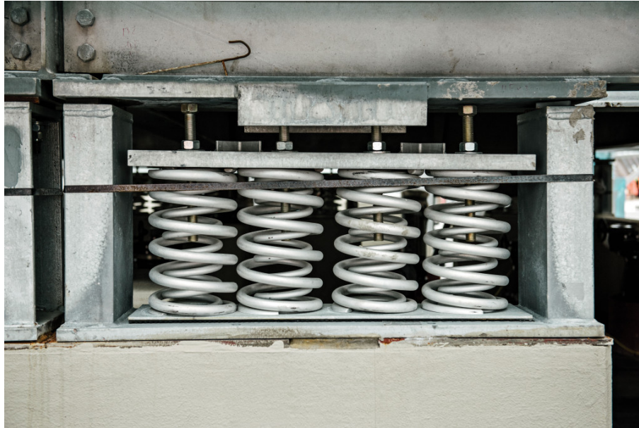
Coils from the cogeneration plant located on the top of the retail complex. Photo courtesy of Joshua Scott
