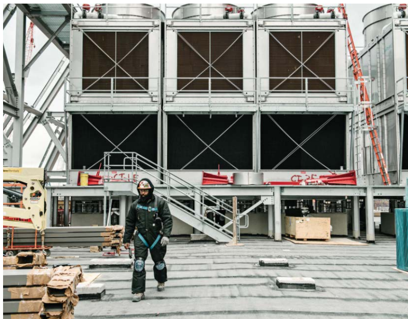
The cogeneration plant on the roof of the retail- restaurant complex. Photo courtesy of Joshua Scott
