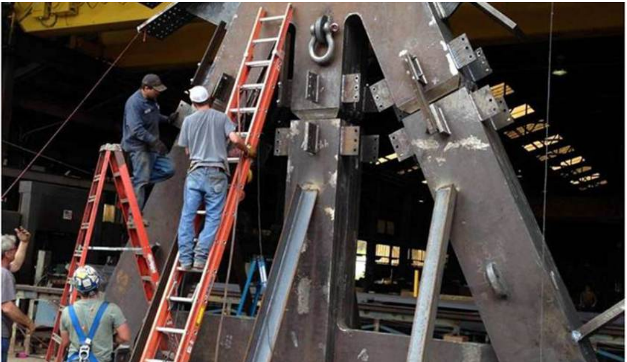
Column used to support the platform of Hudson Yards
